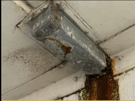
Corroded existing guttering
