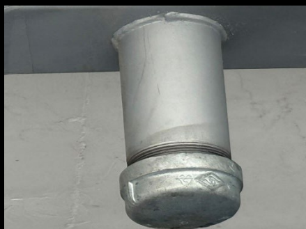
Central drainage point
