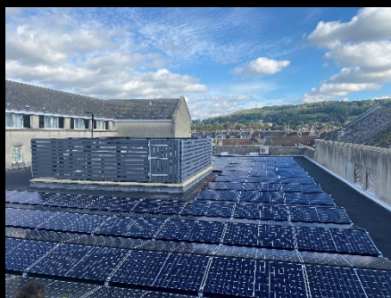
Roof Solar Panels
