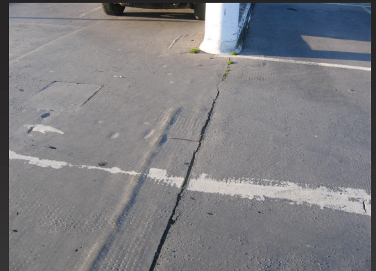
Cracks and repairs in asphalt
